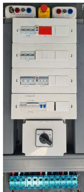
Above: DC wiring side of unit / AC wiring side of three phase unit
